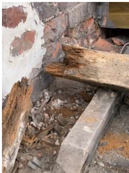
Photo 1 caption: Rotting timbers in the roof structure was a major cause for concern.
